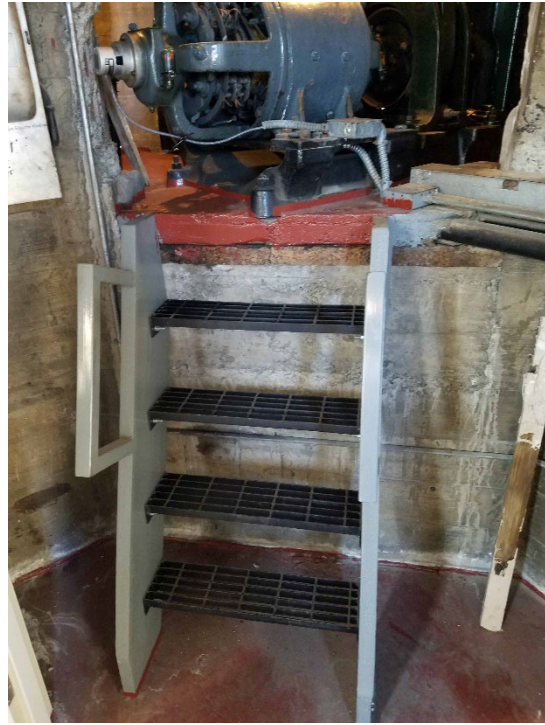
Photo 27: Existing motor above hoistway.
