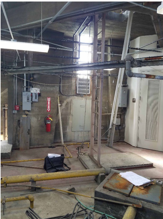
Photo 19: Existing elevator equipment room.
