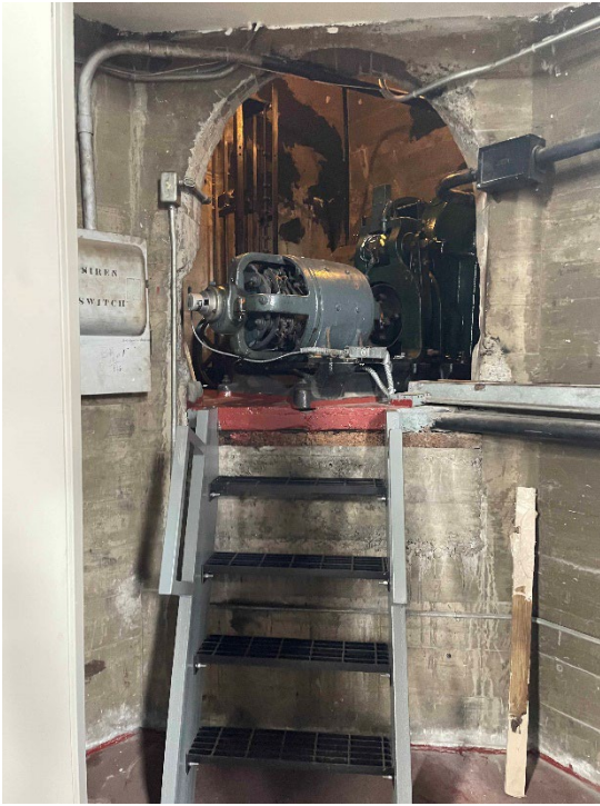
Photo 26: Existing motor above hoistway.
