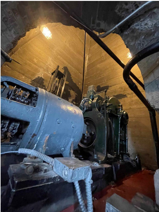
Photo 28: Existing motor above hoistway.
