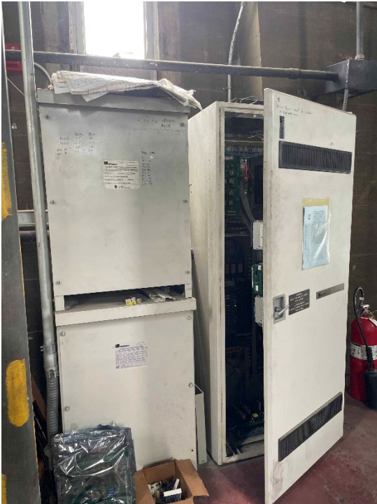
Photo 31: Existing elevator controller.
