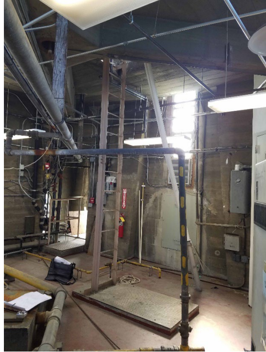
Photo 18: Existing elevator equipment room.
