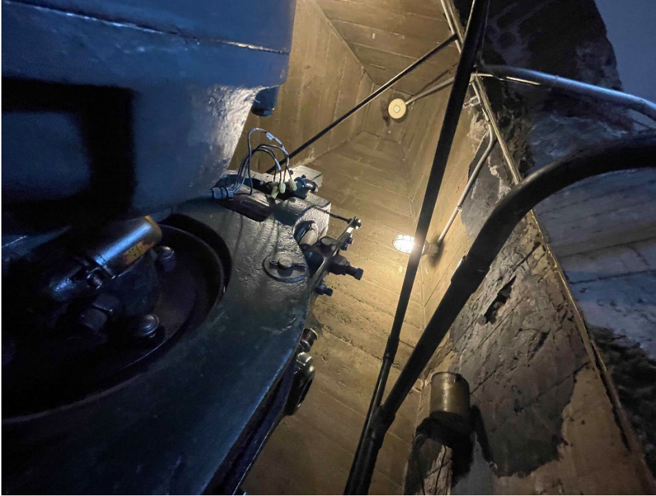
Photo 30: Existing motor above hoistway.
