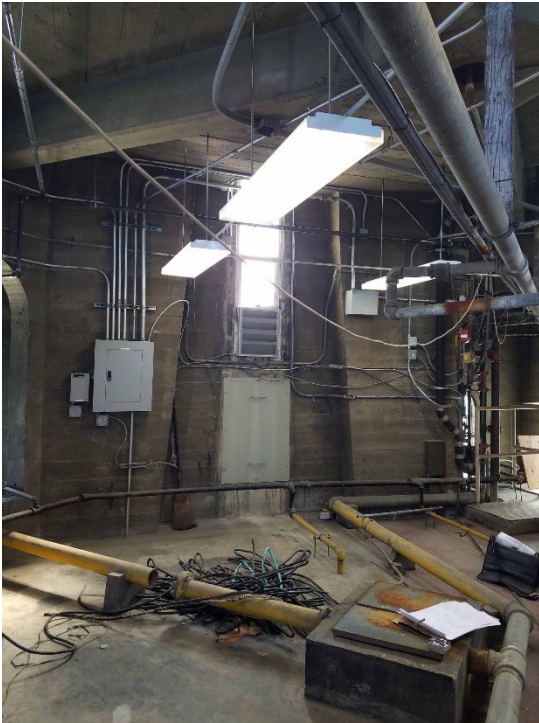
Photo 21: Existing elevator equipment room.
