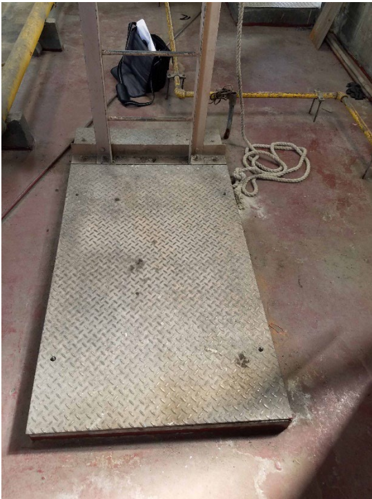
Photo 24: Existing diamond plate cover.
