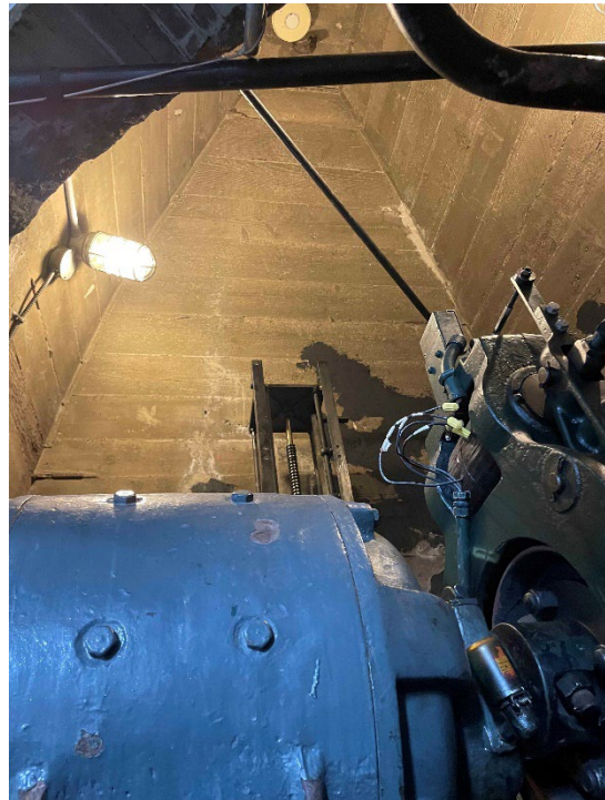
Photo 29: Existing motor above hoistway.
