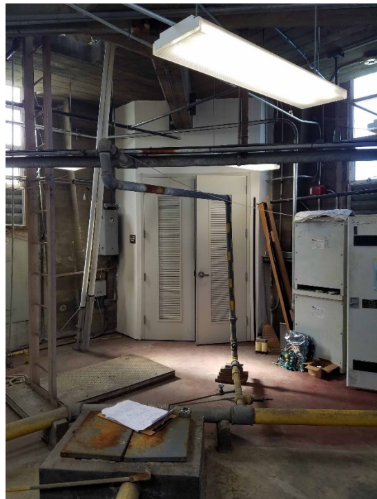
Photo 20: Existing elevator equipment room.
