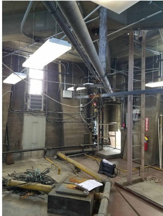
Photo 22: Existing elevator equipment room.
