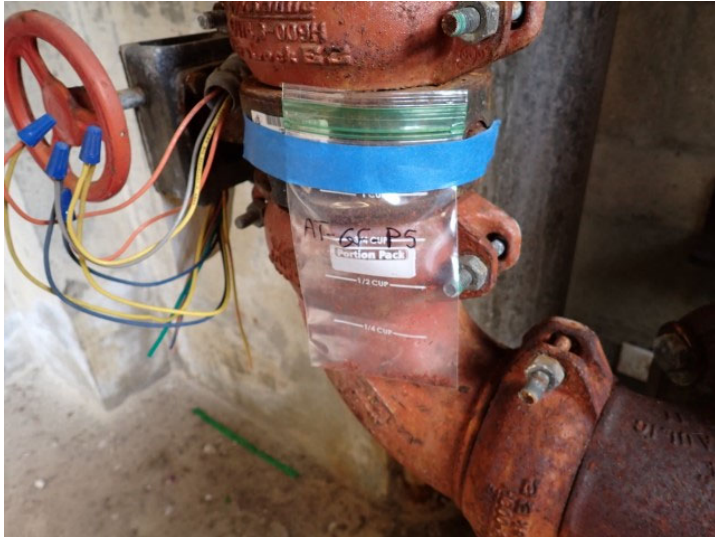
Photo 30 - AT-GF-P05 (Close-Up) [EA\EA162602.JPG]
