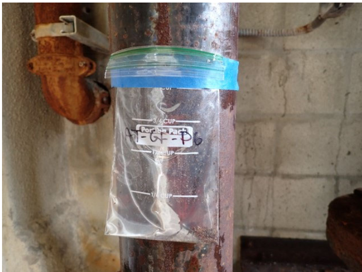
Photo 32 - AT-GF-P06 (Close-Up) [EA\EA162604.JPG]
